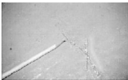
Fig 1 Within 4 hours, subsidence cracks had formed in some of the concrete specimens that didn't contain synthetic fibres
