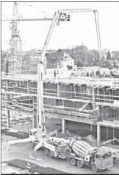
Fig 4 The transit mixer in the foreground discharges concrete into the lorry mounted concrete pump in the background (Note: The articulated telescopic placing boom delivering concrete to the desired location)
