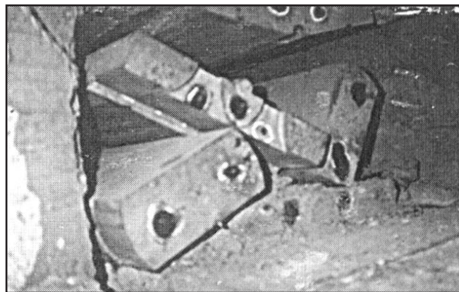
Figure 7. Ramganga bridge - toppled bearing
